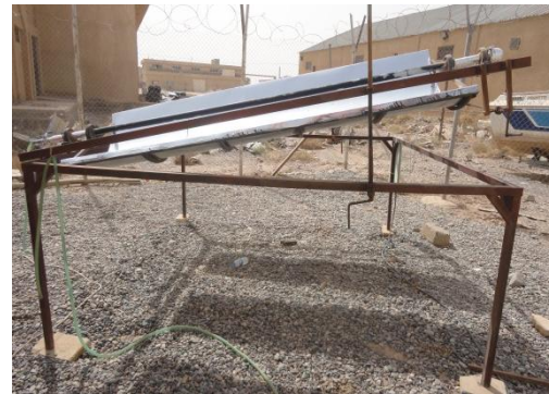
Figure 4b Tracking system of solar concentrator trough
